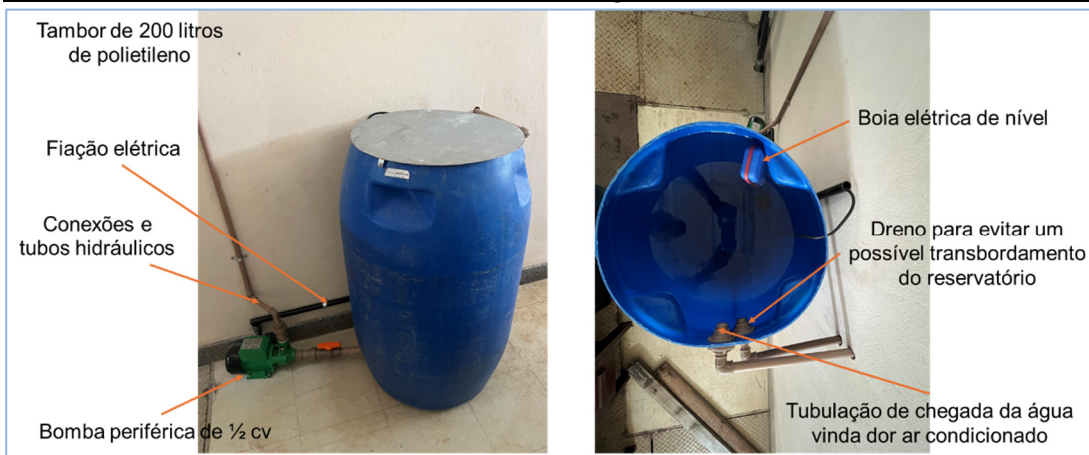
Figure 7: Water collection system from air conditioning system
