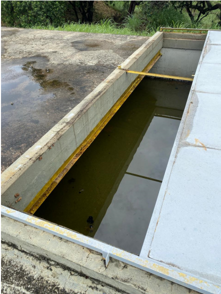
Figure 3: General view of the water and oil separator box.
