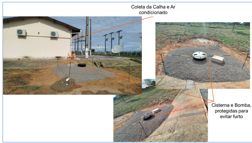
Figure 8: Rainwater and air conditioning collection system
