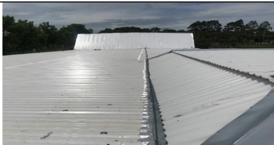
Figure 3: Replacement of fiber cement roofing with thermoacoustic roofing to reduce heat absorption.
